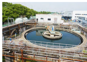
General effluent treatment facilities (Okazaki Plant)
