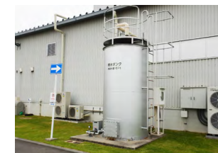
Rainwater storage tanks (Okazaki Plant)
