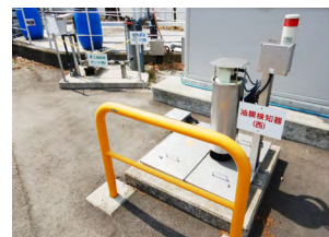
Surface oil detector (Okazaki Plant)
