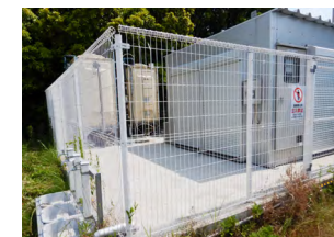
Groundwater membrane filtration equipment (Okazaki Plant)
